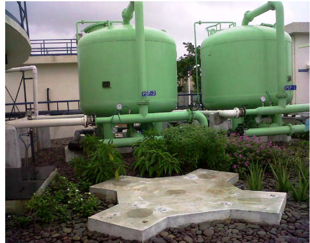
Pressure Sand Filters
